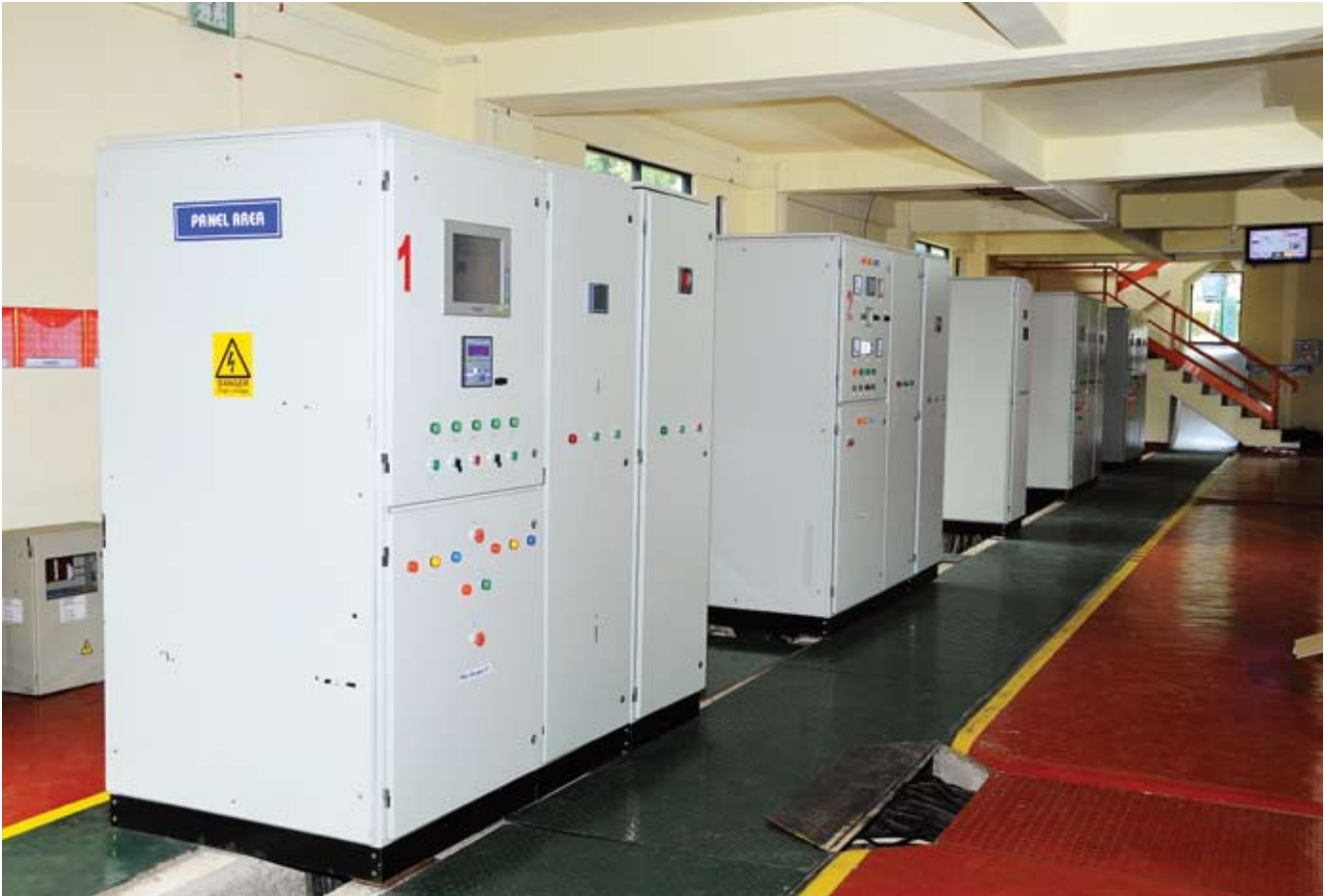
Control Panel Manufactured & Commissioned by Vidul Engineering Ltd.
