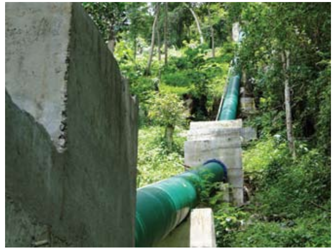
Penstock - Ganthuna MHPP
