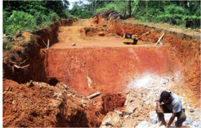
Forebay location at Wembiyagoda MHPP
