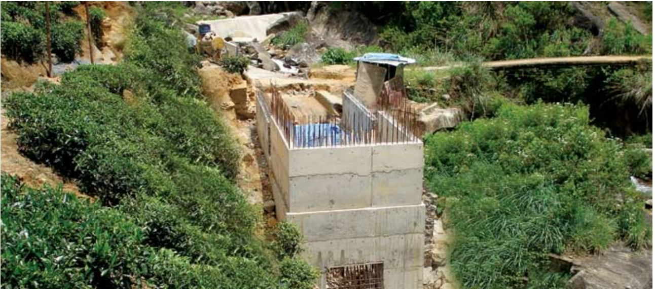
Construction work proceed at the Fore bay Tank – Sheen Mini Hydro Power Project
