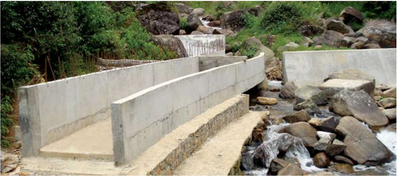
A Section of the Head Race Channel – Sheen Mini Hydro Power Project
