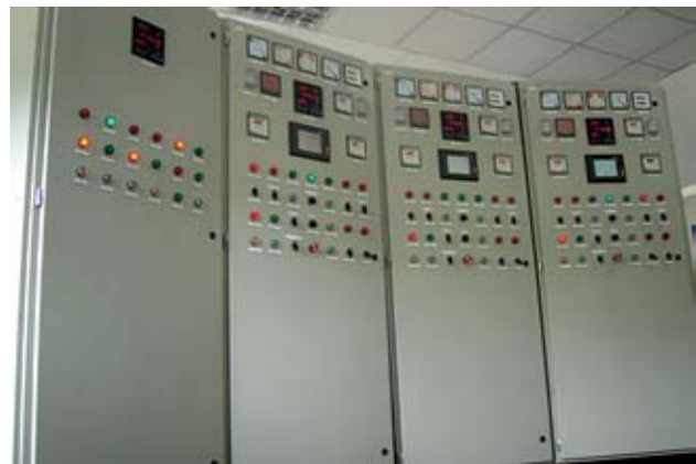
Synchronised Panel board – Batatota Plant
