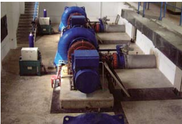
Turbines in operation – Batatota Plant
