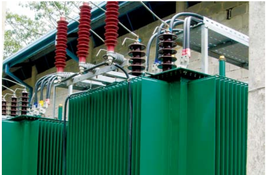
Step-up Transformers - switchyard - Batatota Plant
