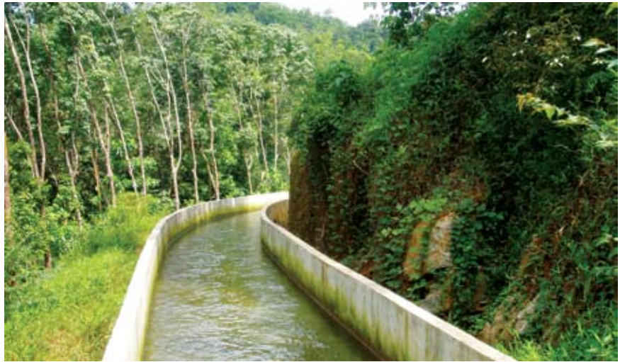
A section of the Head Race Channel - Batatota Plant
