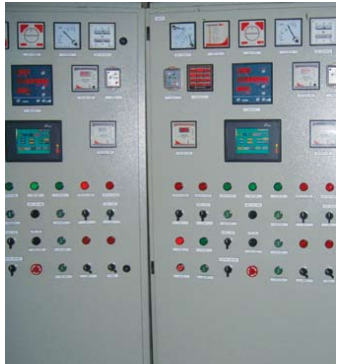
Control Panels - Batatota Plant
