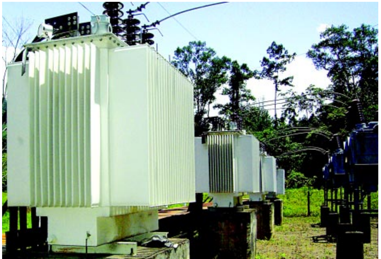
A View of the Transformers
