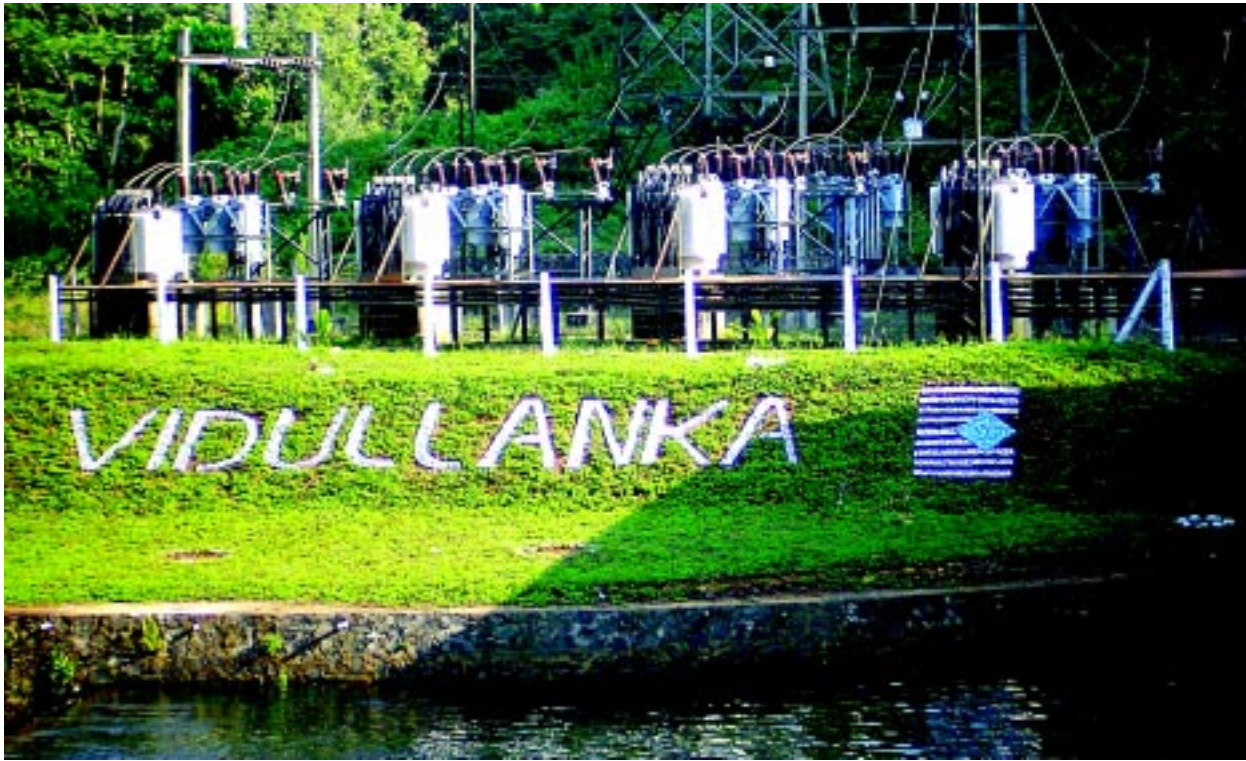
A view of the Switch Yard
