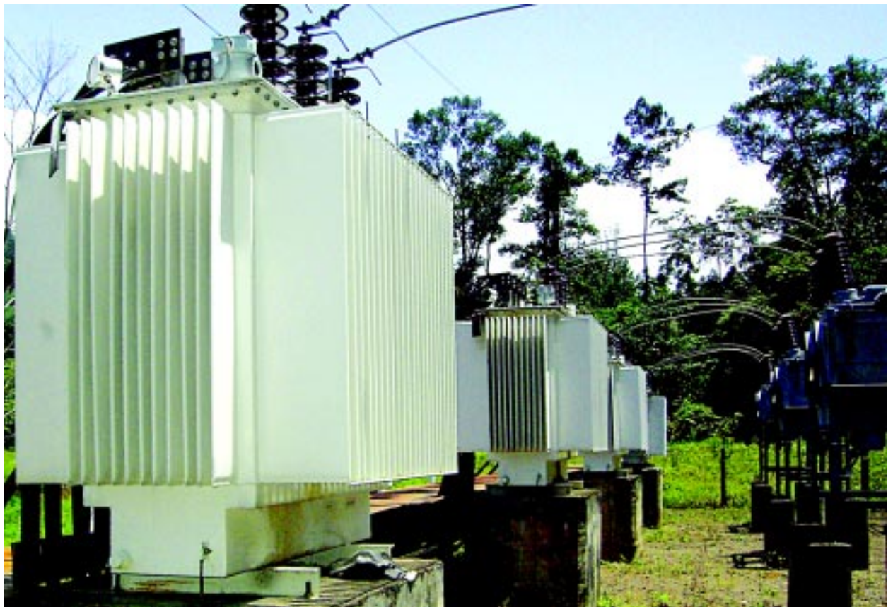
A View of the Transformers
