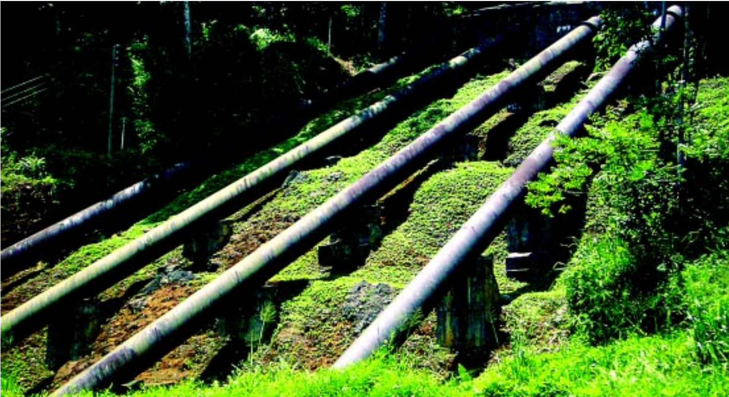
A View of the Penstocks
