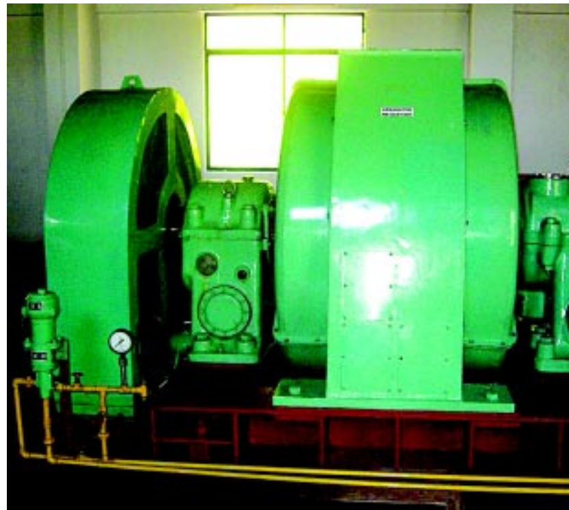
A view of the Generator
