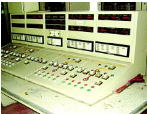
The Main control panel
