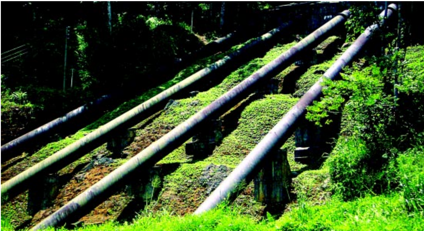
A View of the Penstocks
