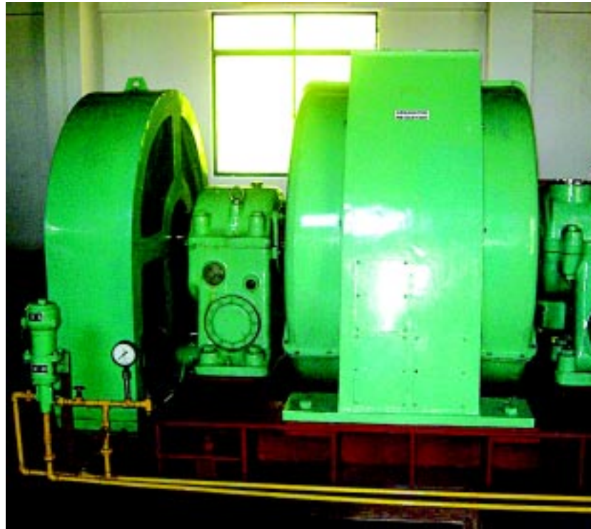
A view of the Generator
