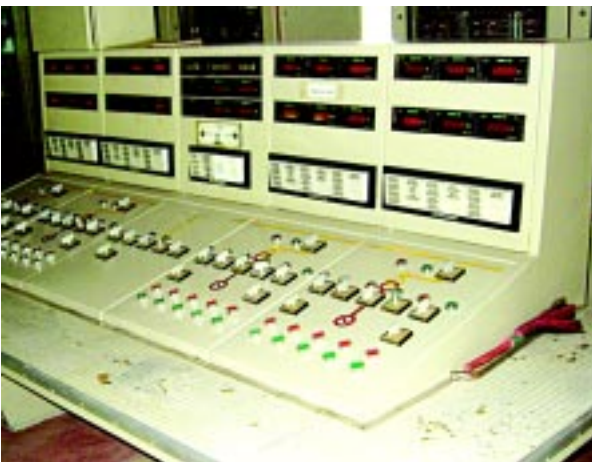
The Main control panel
